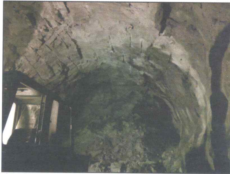
Fig. 5 Tunnel profile with minimum overbreak after application of new blasting techniques at LNPHEPP
